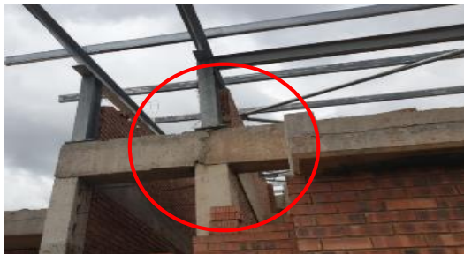
Nursing college – defects in concrete beams causing cracks
