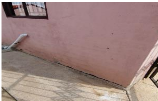
Foundation and brickwork defects causing water seepage into house
