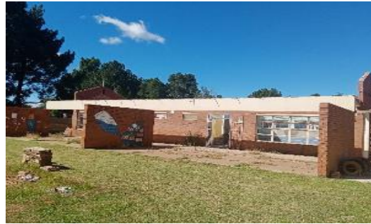
Stripped grade R classroom – refurbishment delayed
