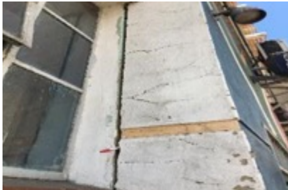
Police station – cracked column
