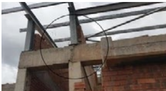
Concrete beams cast separately in parts, with visible cracks and concrete overlap in attempt to repair cracks
