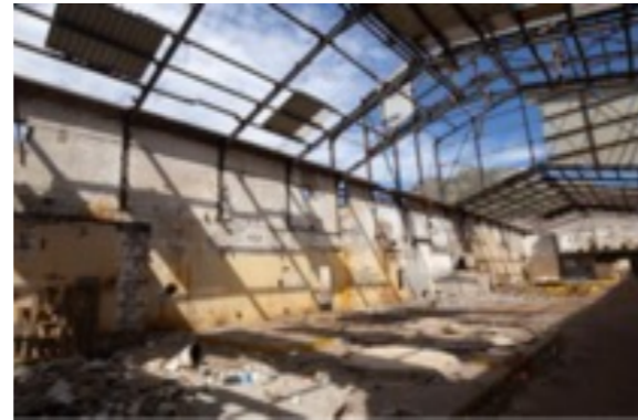
Fishmeal factory – abandoned and stripped by looters
