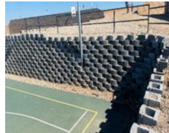
Top retaining wall blocks loose
