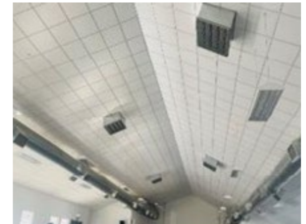
Leaks around ventilation units due to poor waterproofing
